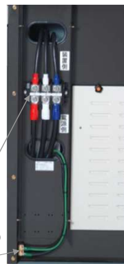
Ground terminal block (lower side = customer wiring side)
